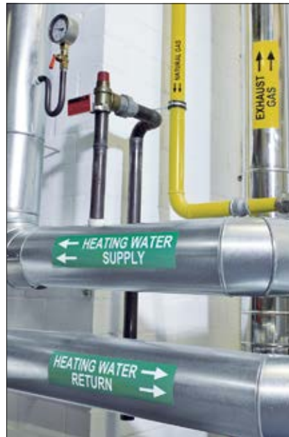
Large and highly visible pipe marking.
